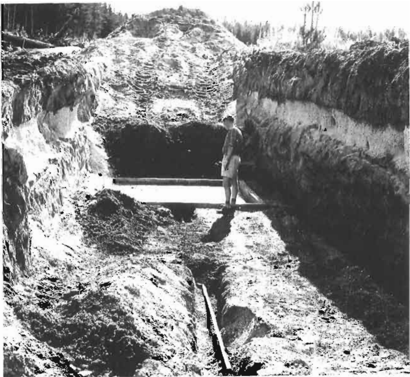
FIG. 4—Lysimeter collection pad and drainage pipe at base of excavated trench before replacement of soil profile.
